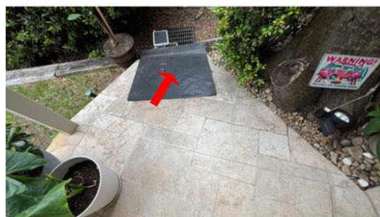
Potential slip hazard when wet
