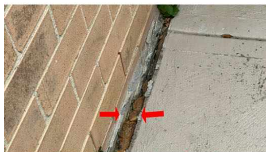
Detached from wall considerably
