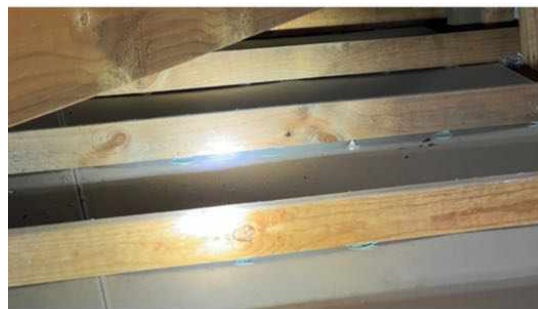
Ceilings detached from joist throughout garage
